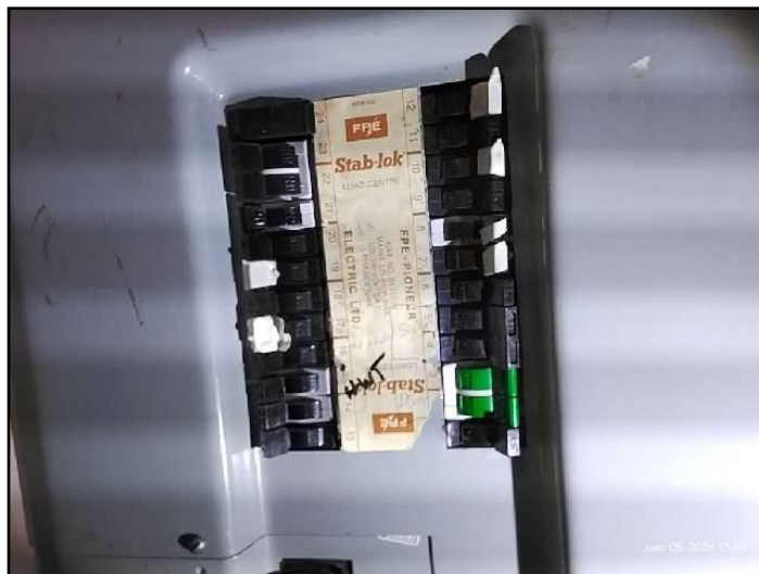
17. Breakers - utility room
