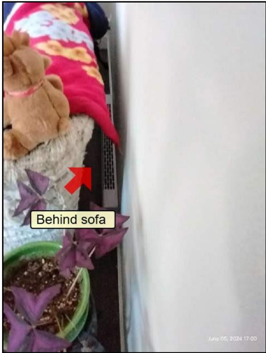
41. Noted few things on baseboard heater in...
