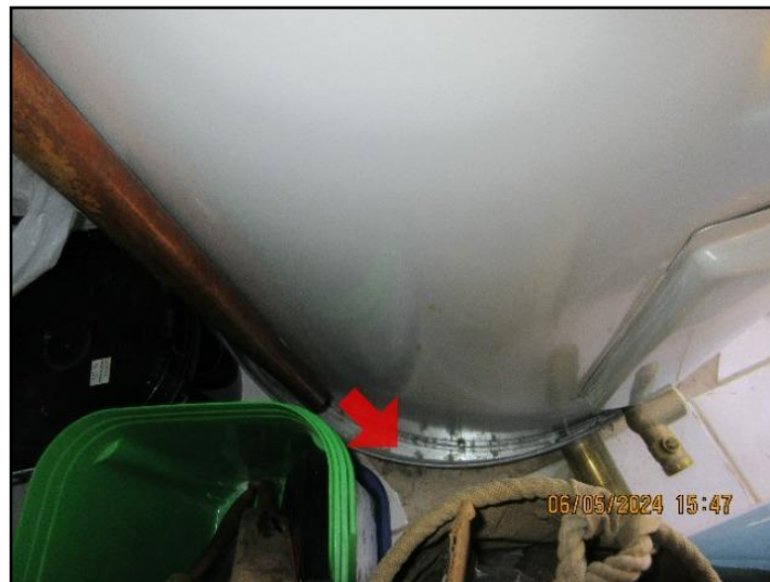
53. Water heater drain pan
