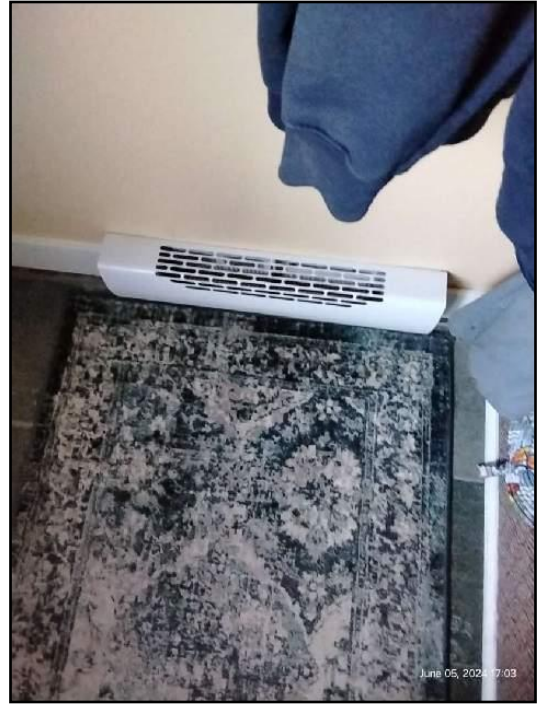
34. Electric baseboard heaters Thermographer...
