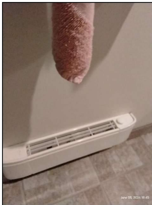
32. Electric baseboard heaters Thermographer...
