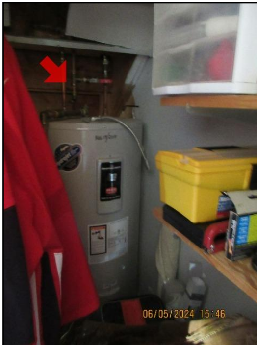
56. TERV: No expansion tank has been installed...
