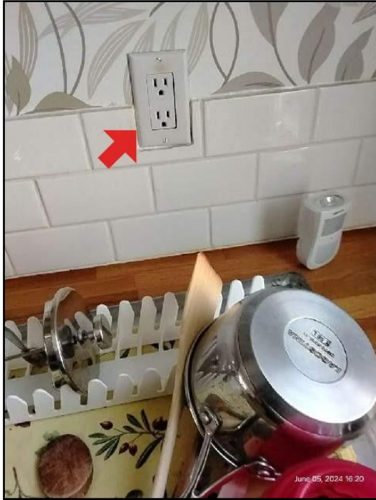
20. No GFCI in kitchen
