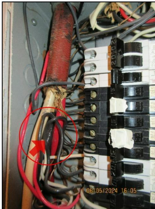
28. Not well secured
