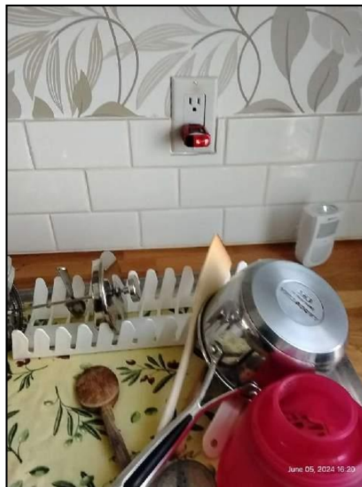
29. No GFCI/GFI (Ground Fault Circuit...
