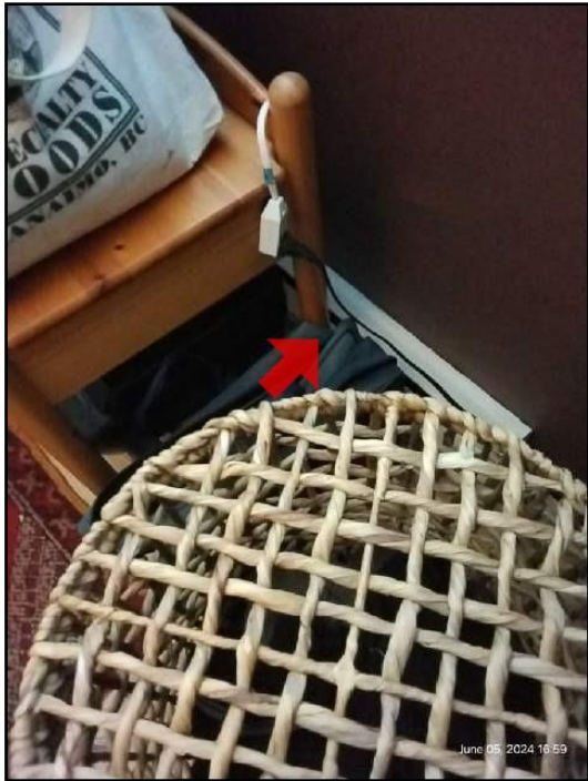
40. Noted few things on baseboard heater in...
