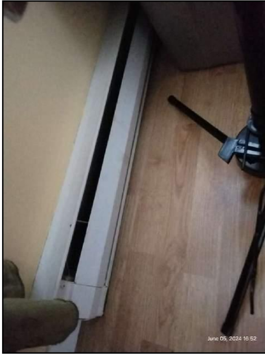
33. Electric baseboard heaters Thermographer...
