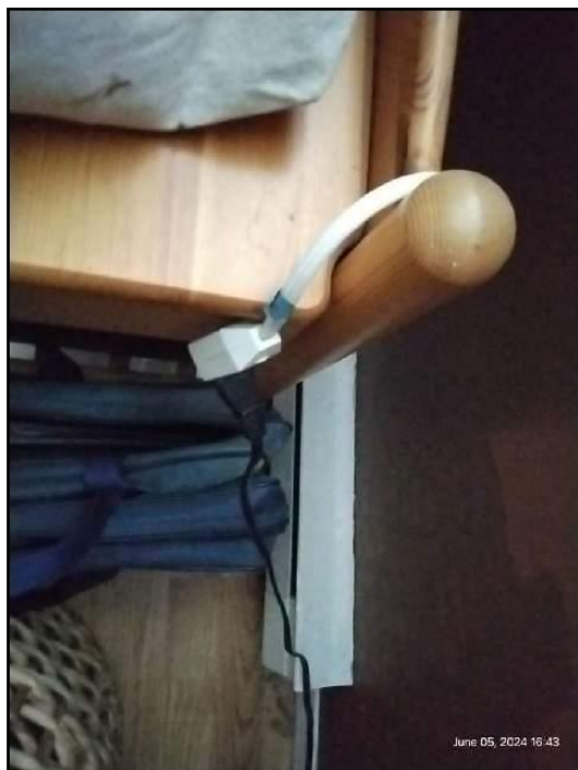
31. Electric baseboard heaters Thermographer...
