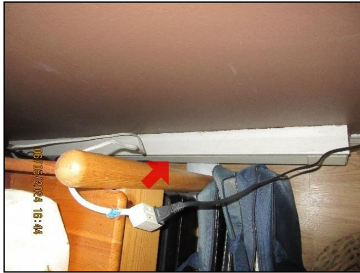
42. Noted few things on baseboard heater in...
