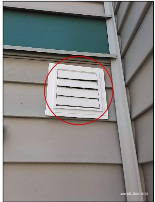
75. Range hood discharges to the exterior
