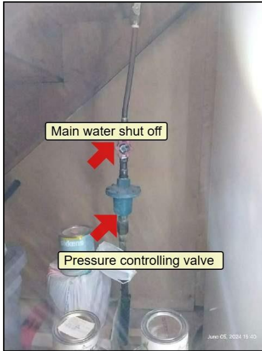
44. Near water heater
