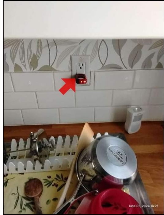
21. No GFCI in kitchen
