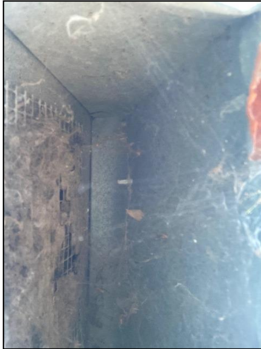
68. fresh air intake clogged
