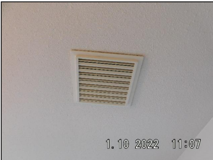
105. Exhaust fan bathroom 1
